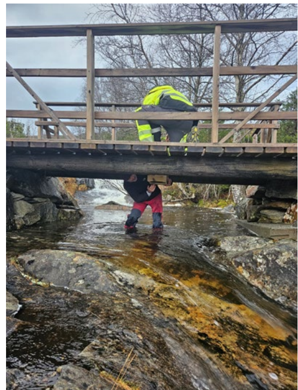
Installation of hatching boxes under a side river bridge. Photo: Marianne Kanstad
